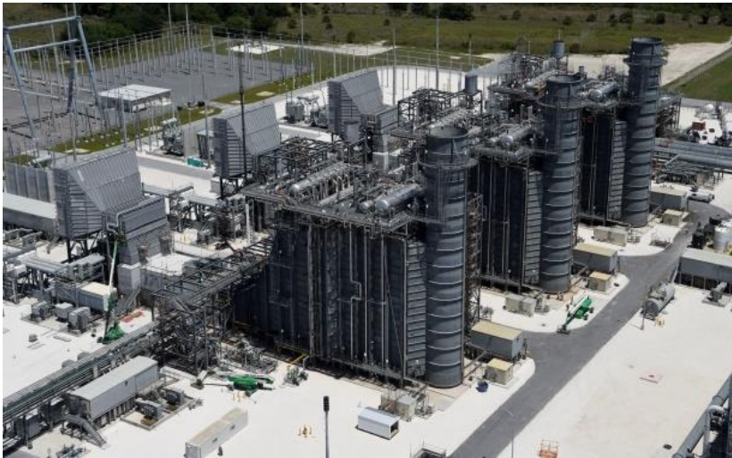
FPL's Okeechobee Clean Energy Center COD March 2019
